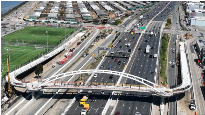
Bicycle and pedestrian overcrossing that is Phase 1 of the I-80 Gilman Interchange Improvement project.
