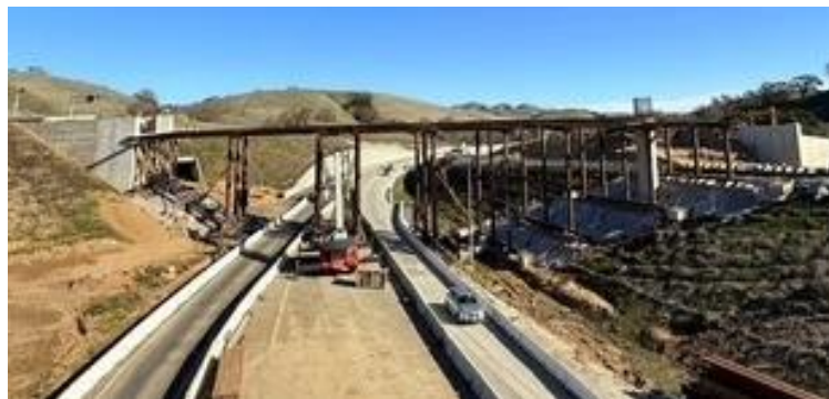
Crews prepare to construct the flyover bridge at the northbound I-680 Calaveras on-ramp.
