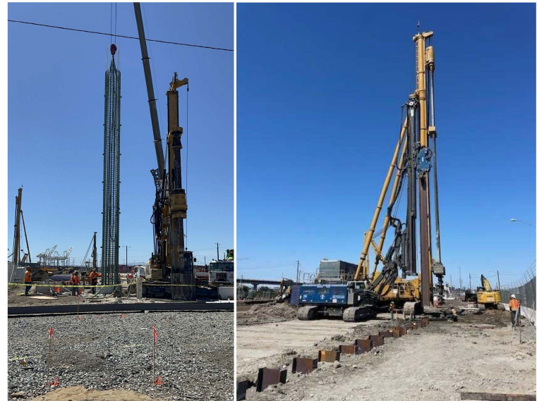
(Right) Steel reinforcement cage installation and (Left) Steel beam piles are driven into the ground in preparation for excavation of new roadway and bridge.
