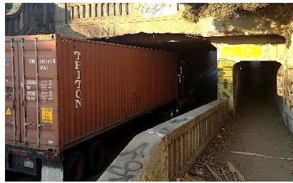
Existing multi-use path and damage to the 7th Street underpass.
