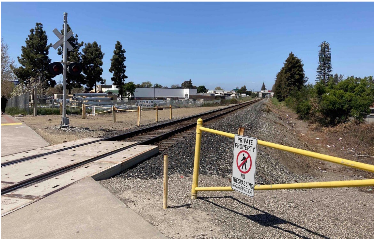
Photograph 16. View of railroad tracks and safety measures to be improved north of the crossing at Lewelling Boulevard, facing west-northwest.
