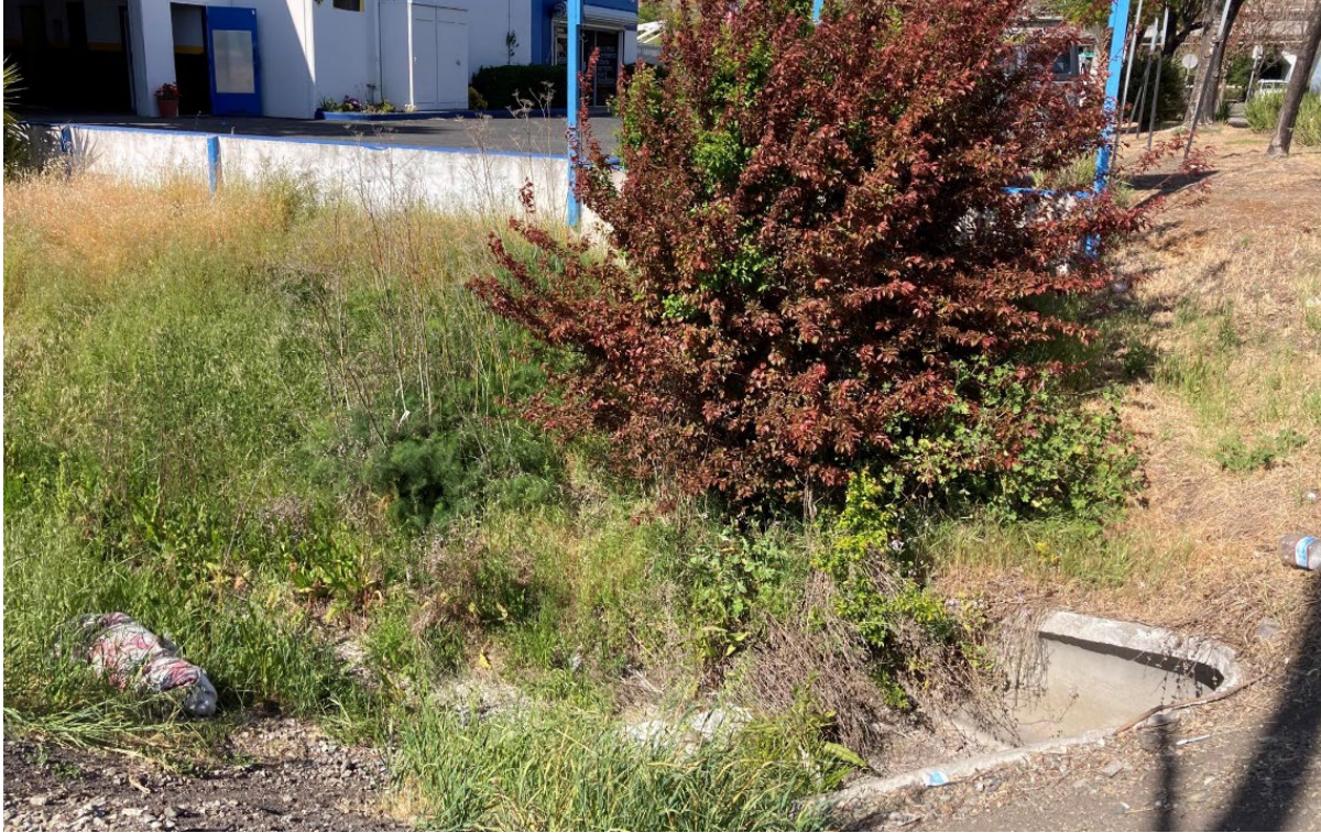
Photograph 31. View of culvert that connects drainage ditch on northwest side of Industrial Parkway to Ward Creek on the southeast side of Industrial Parkway, facing north.
