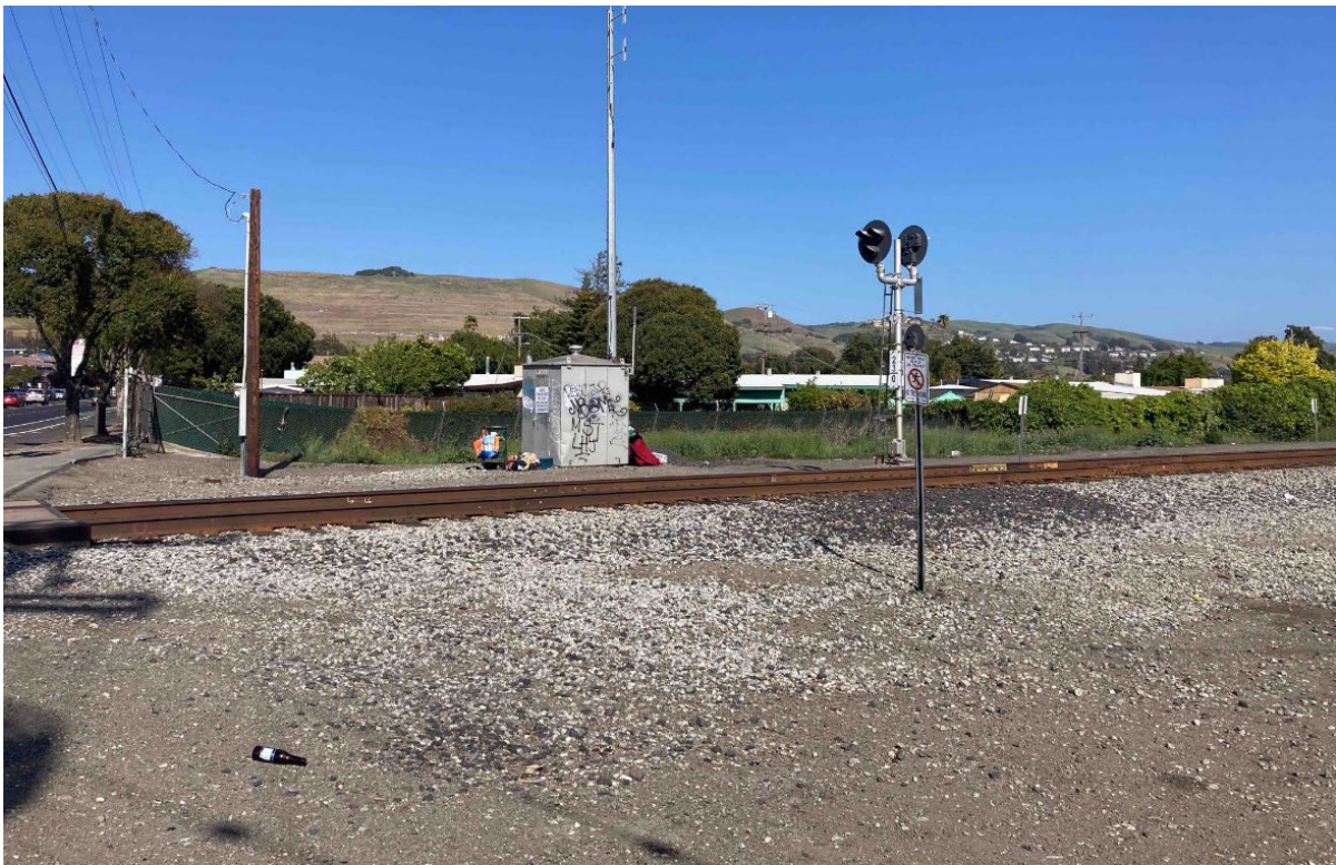
Photograph 26. View of railroad tracks to the south of the Tennyson Road crossing, facing east-northeast. A drainage ditch occurs along to the east of the tracks.
