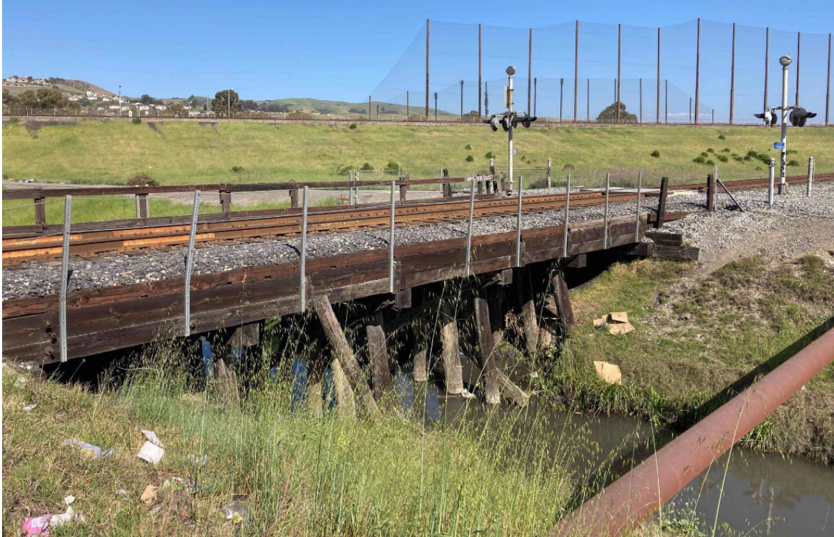
Photograph 33. View of bridge over Ward Creek and pedestrian crossing for trail to the southeast of Industrial Parkway railroad crossing, facing northeast.
