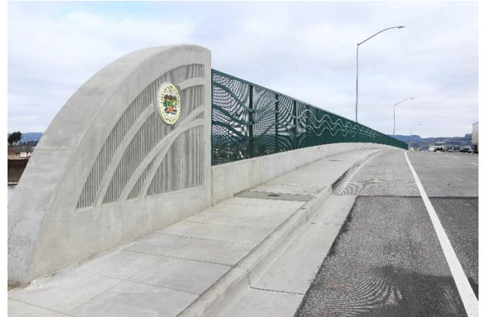
Decorative end corbel with green bridge railing, Courtesy of the California Department of Transportation
