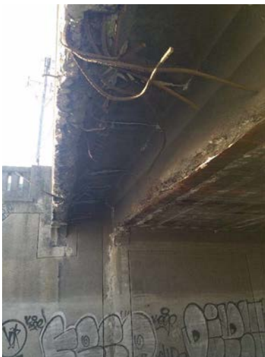
Figure 2: Truck strike damage at bridge
