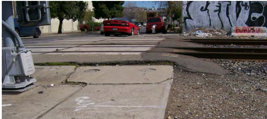
Tripping hazard in sidewalk
