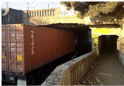
Existing multi-use path and damage to the 7th Street underpass.
