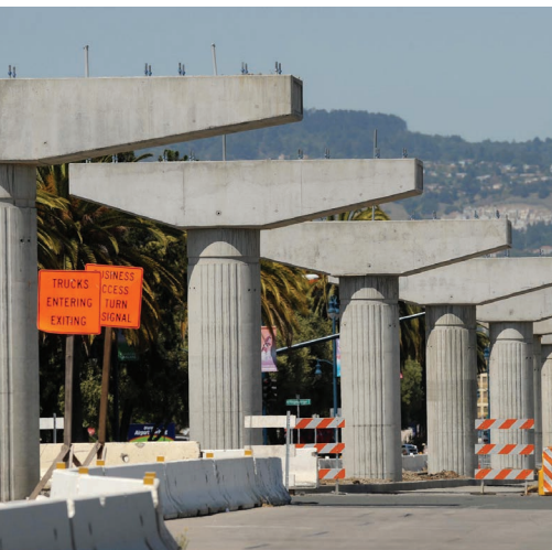
Measure B funds 18 percent of the $484 million BART Oakland Airport Connector project that will improve transit choices and connections for travelers to and from the region.
