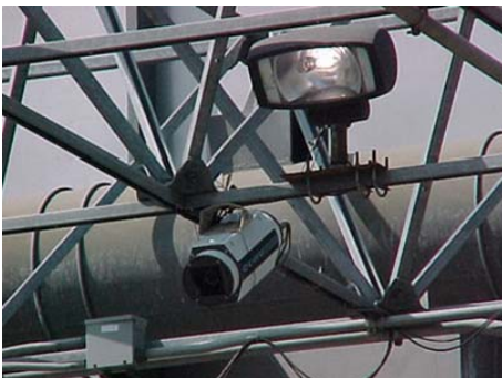
Figure 4: Example of Camera and Flash Light used in Automated Violation Enforcement
