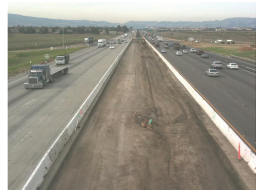
Construction is underway to provide an HOV lane on Interstate 580 between Livermore and Pleasanton, a project to help ease the commute congestion.
