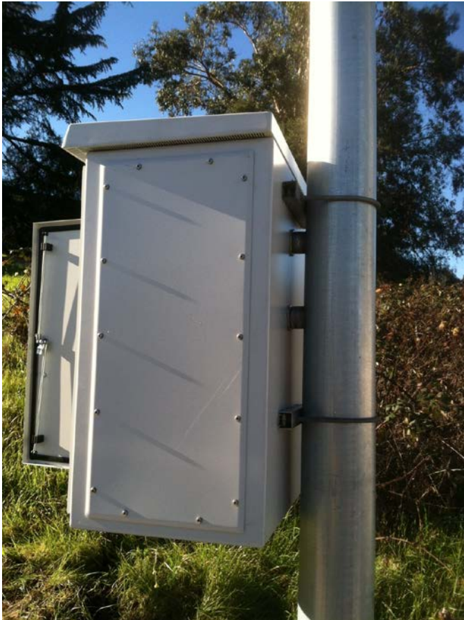
CCTV Cabinet – Various Locations
