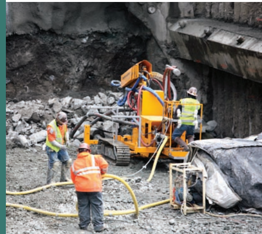
Caldecott Fourth Bore Project located on State Route 24 between the cities of Oakland and Orinda.
